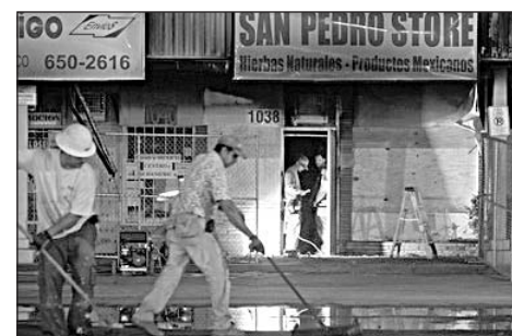
Cleaning up after fire
